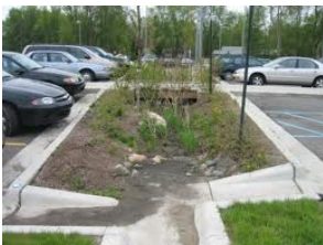
Parking lot rain gardens are a sustainable approach to managing stormwater runoff.
